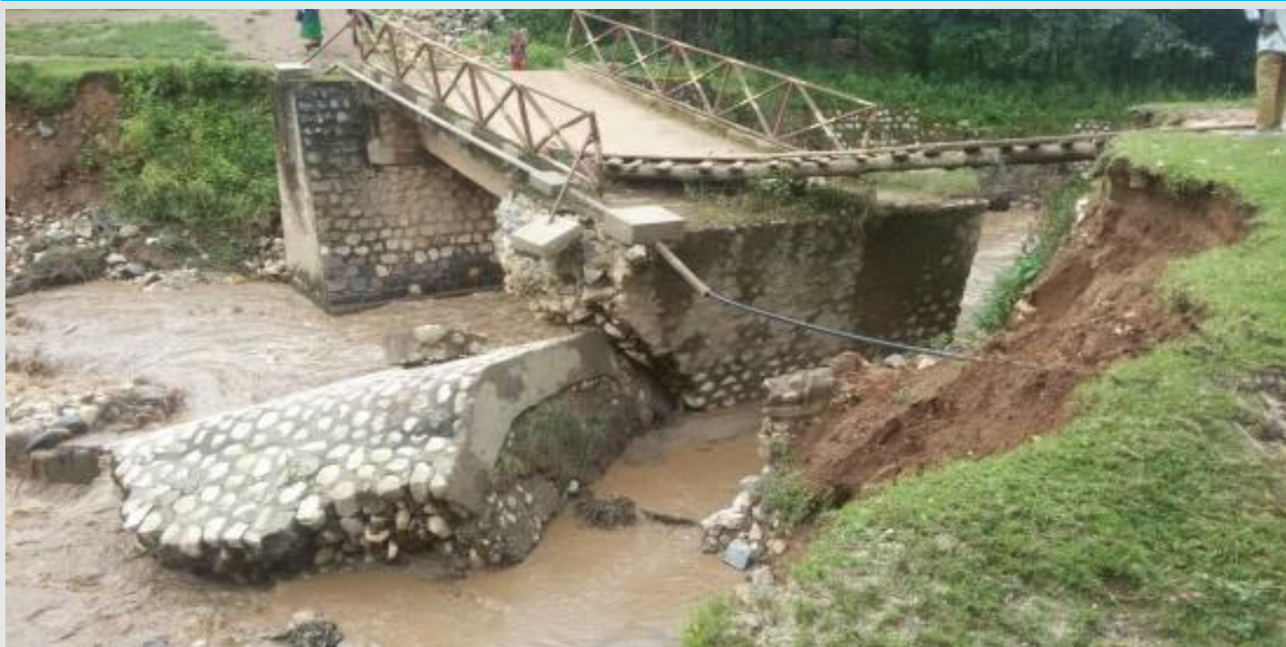
Gatare Bridge collapsed
